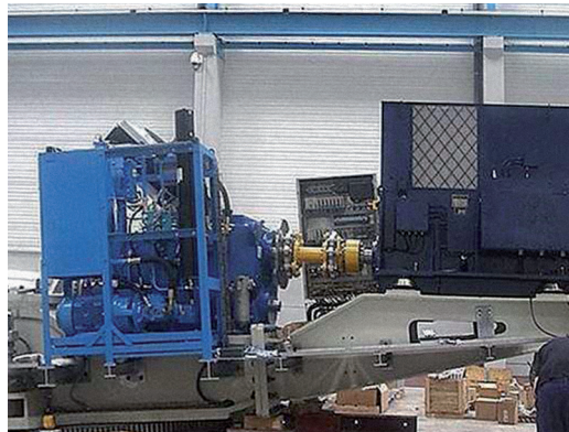
IXILFLEX coupling in wind turbine.
